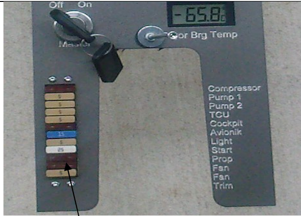
Fuse location on instrument panel (second from bottom position)
