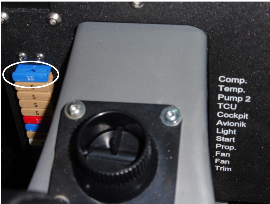
Fig. 2: 15A Fuse Compressor
