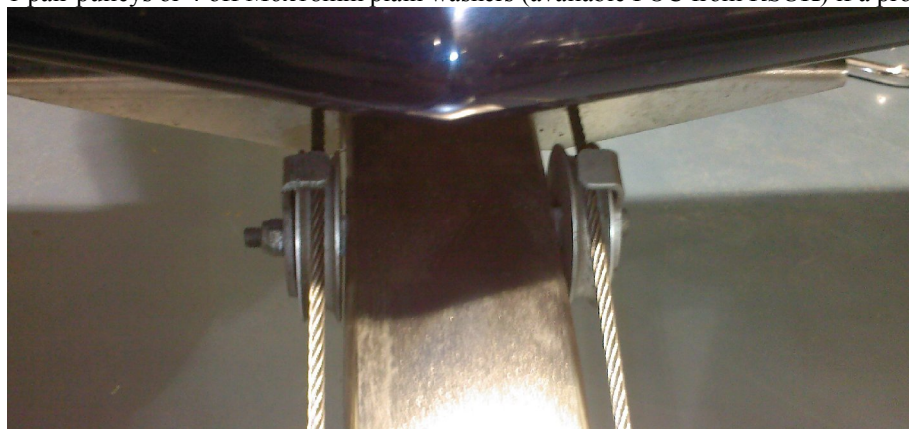
Picture of rear rudder cable pulleys
