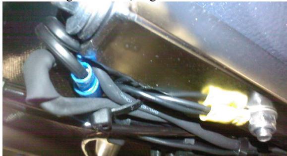
View of underside of left bolt, showing earth cable.
