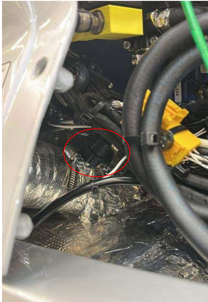
Figure 9 – Fuel vent hose LH fuel tank
