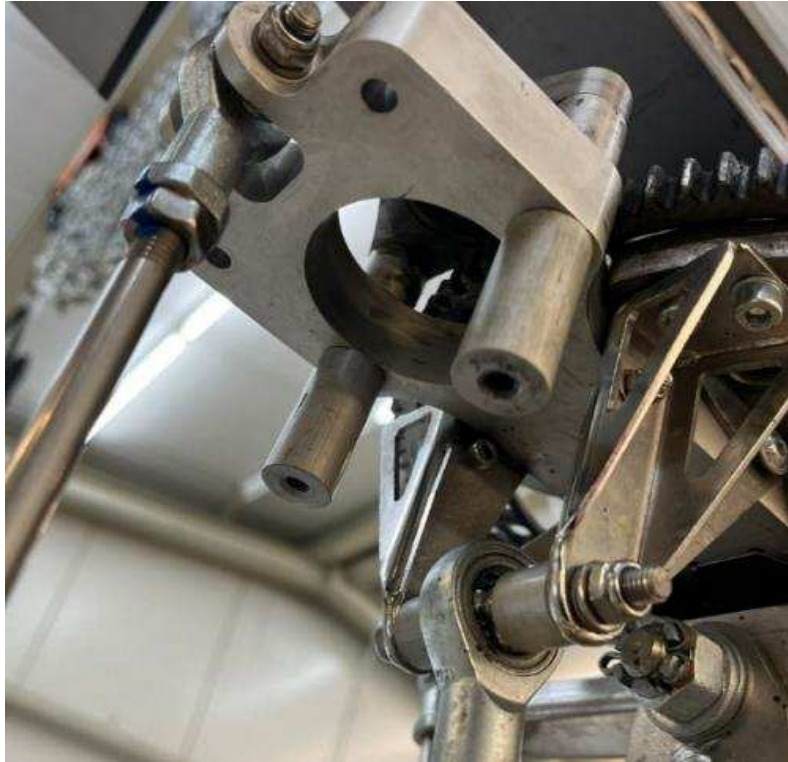
Figure 5 – Lower bearing mount removed from rotor head
