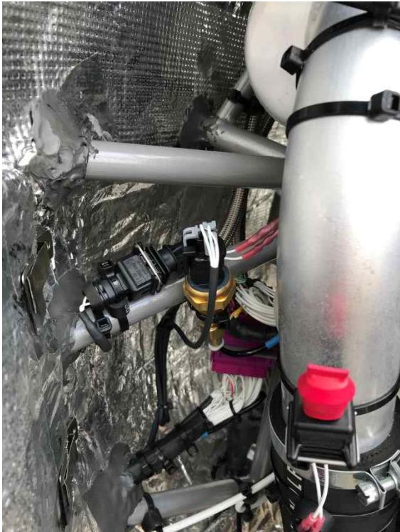
Manifold pressure sensor located in engine bay (attached to engine frame)
