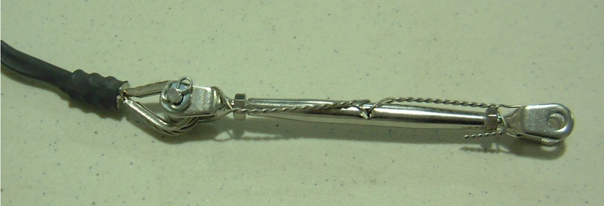
Acceptable wire locking of turnbuckle
