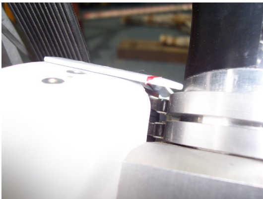
Picture showing pitch limit switches running on blade cams
