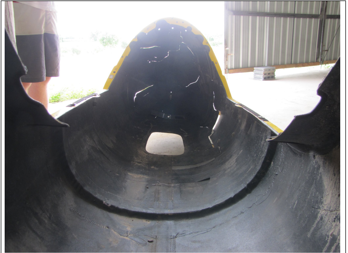
View inside before repair. From this and the other photos it can be seen that the attachment points to the airframe are sound, and that the damage is limited to the nose section only.
