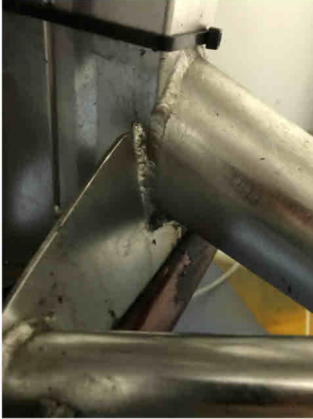
View of the bracket to mast weld area on the first UK Calidus frame. Note that the bracket is welded to the mast, not to the keel tube.
