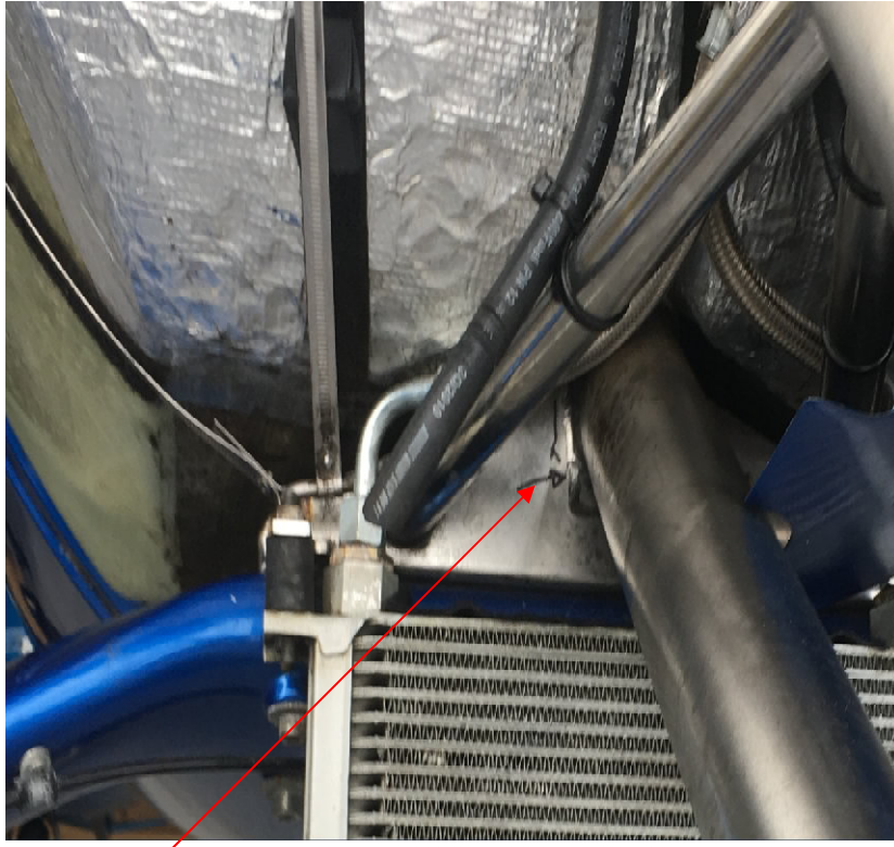
Crack position for SRA-023 (could be either side of the mast)
