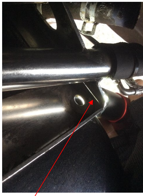
Crack position for this SRA-024 (mounting bolt removed and illuminated from rear)
