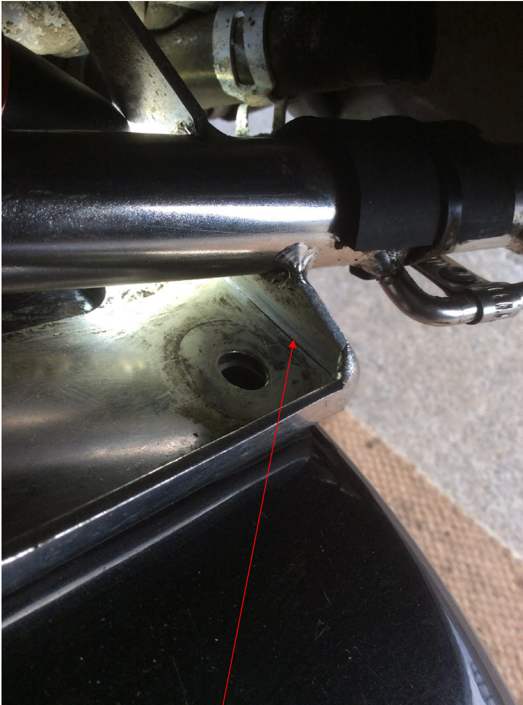
Magnified view of crack for this SRA-024
